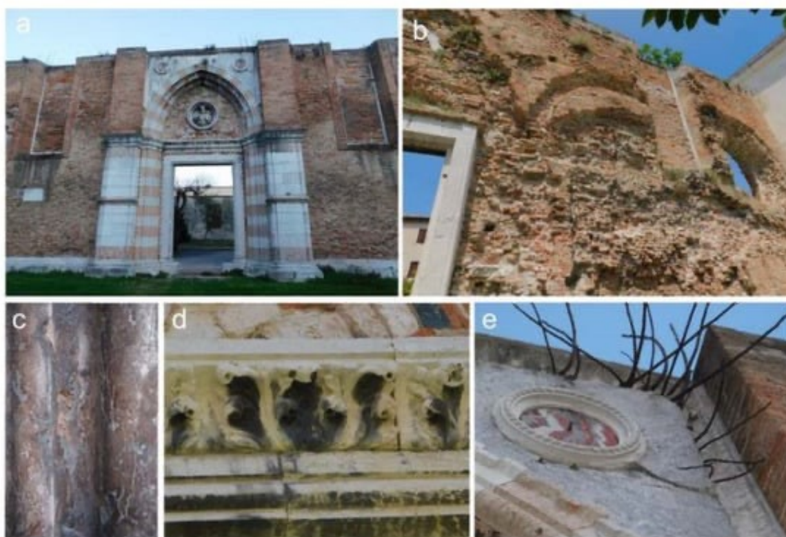
Figure 17: Details of the main façade of the ruins of Santa Maria dei Servi Church: (a) the external main portal; (b) the internal main portal; (c) exfoliation of red Verona marble used in the portal; (d) detail of ornamental Istrian stone use in the portal with black crusts in sheltered areas; (e) detail with Proconnesian marble (grey) and the tondo in Cipollino marble (red); secondary plants ( figus carica ) growth is also visible.
