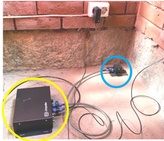
Figure 4: Test setup for Ambient Vibration Testing: the accelerometer and the data logger are identified in blue and yellow circles, respectively
