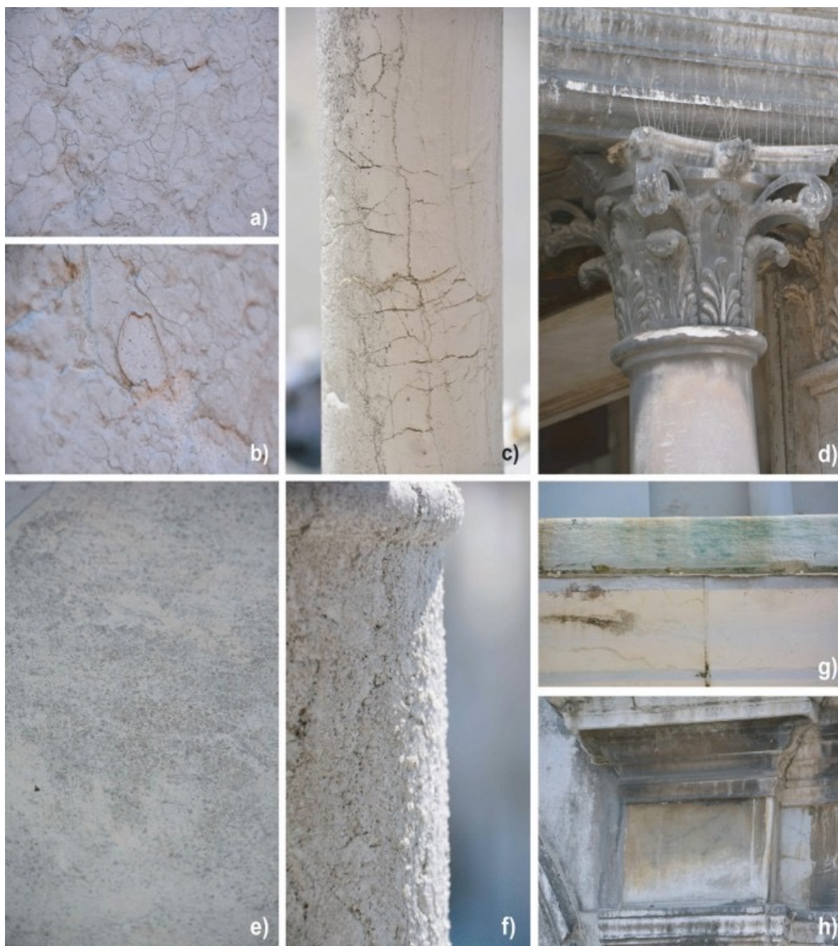
Figure 15: Features induced by material loss: a, b differential erosion on Ammonitico Rosso from Verona slabs (eastern façade), c microkarst on Istrian Stone small columns (western façade). Discoloration and deposit: d black crusts on Istrian-stone Corinthian capitals (southern façade); e soiling on Scaglia Rossa slabs (western façade); f efflorescence on Istrian Stone small columns (western façade); g greenish staining on Istrian Stone (western façade); h yellowish patinas (southern façade)
