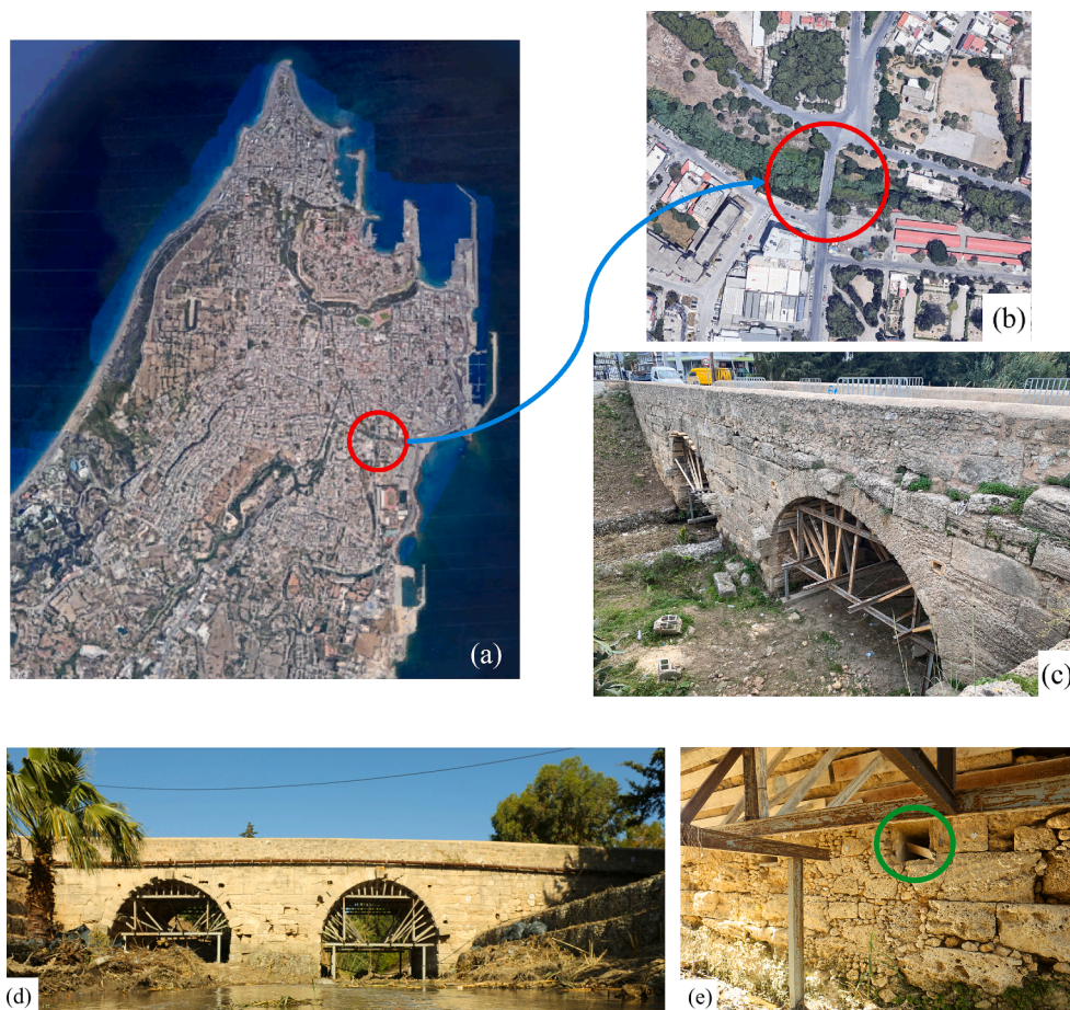
Fig. 2. (a) Rhodes Island in Greece and location of the Roman bridge, (b) top view of the Roman bridge, (c) and (d) Roman bridge from different views, and (e) holes in the central pier with erosion.
