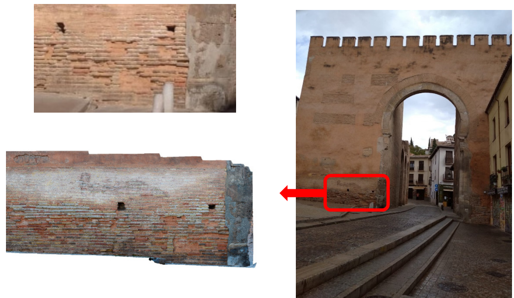
Figure 5. Detail of the restoration work carried out with bricks on the east façade of Puerta Elvira.
