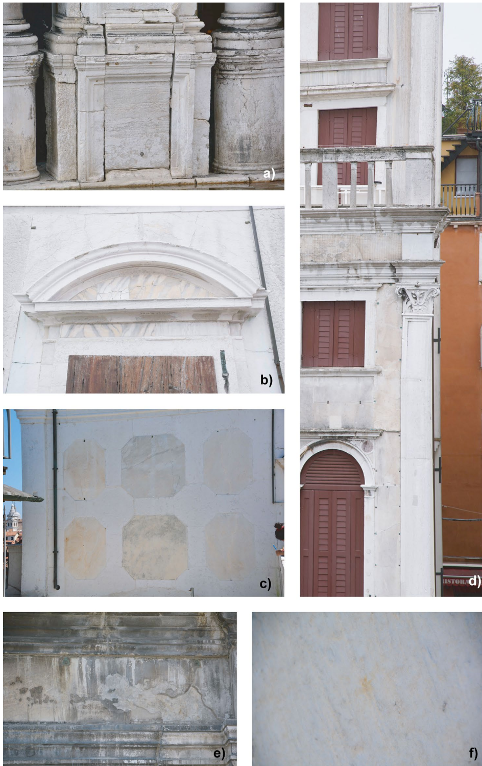
Fig. 4 Crack and deformation: a fractures on a pillar base (southern façade), and b on the marble slabs decorating the doorframe arch (eastern façade); c faint convex deformation on marble slabs (western façade); d lestone deformation (southern façade). Detachment: e blistering phenomena (southern façade); f sugaring phenomena on marble slabs (western façade)
